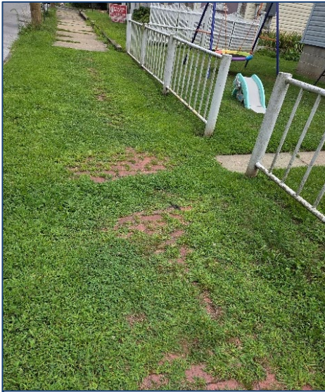
Figure 3: Example rough sidewalk condition
